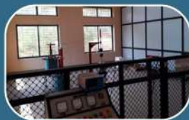
POWER SYSTEMS LABORATORY
